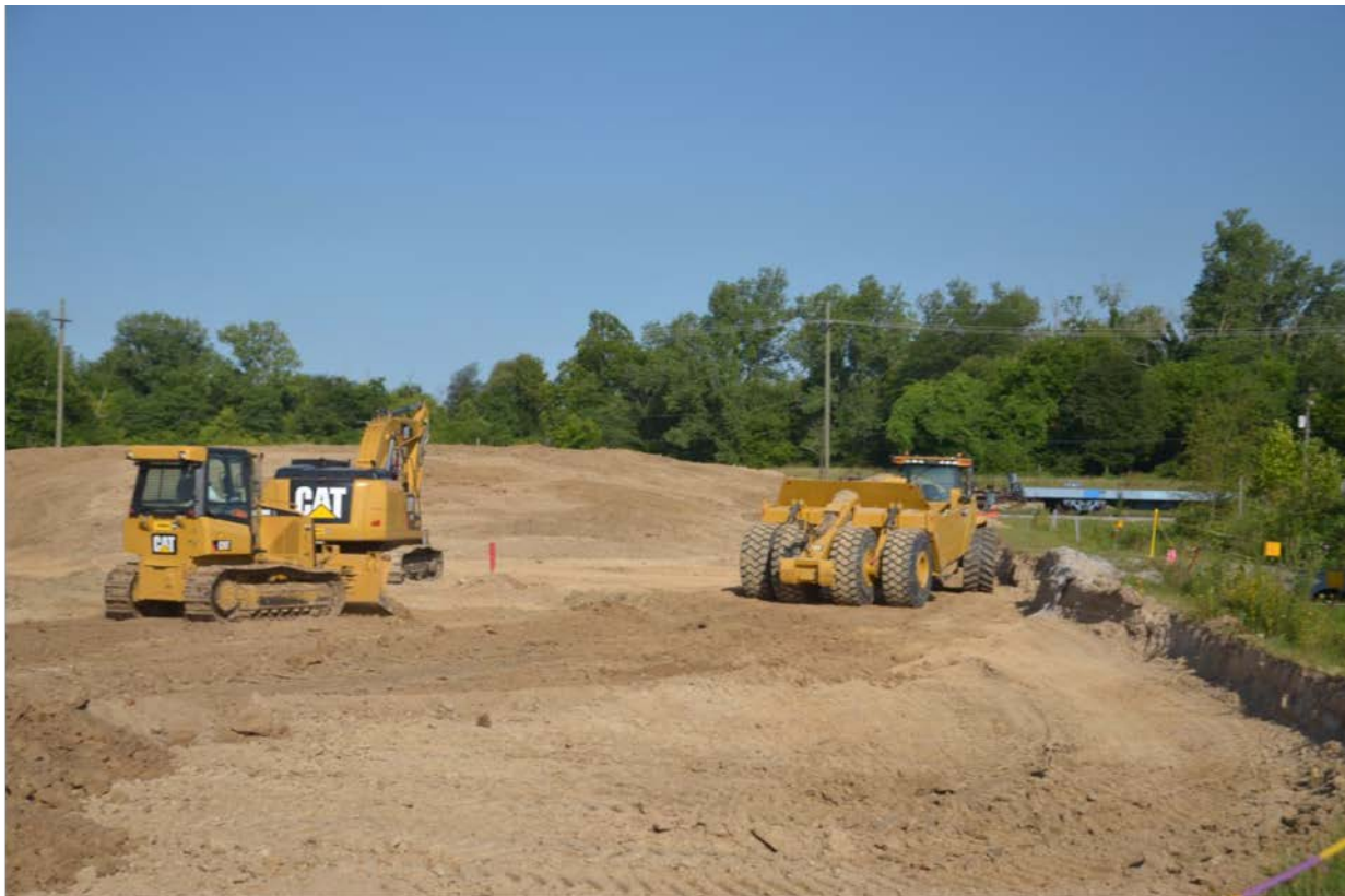
Figure 6.6 Remedy implementation at SWMU 1, a former oil landfarm and source of TCE groundwater contamination to the Southwest Plume.
