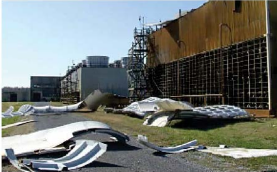
Figure 3.1 Cooling Tower Damage from the 2013 tornado.
