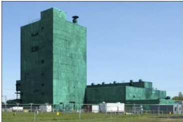
Figure 17. C-340 Metals Complex with transite siding that is sealed to stabilize hazardous and radioactive materials during demolition
