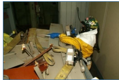
Figure 22. Deactivation radiation screening
