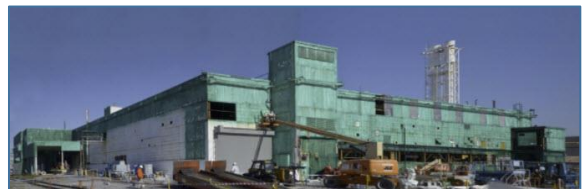
Figure 21. C-410 & C-420 Complex
