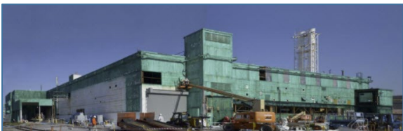
Figure 21. C-410 & C-420 Complex
