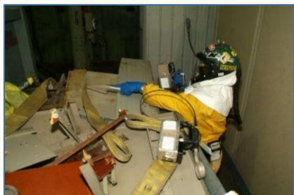
Figure 22. Deactivation radiation screening
