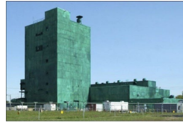
Figure 17. C-340 Metals Complex with transite siding that is sealed to stabilize hazardous materials and asbestos during demolition
